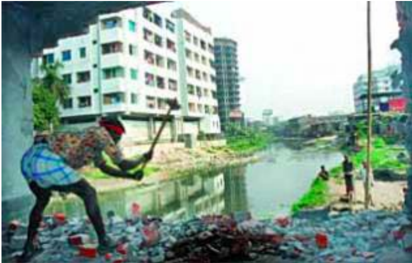
Demolition of an unauthorised structure on the Kalyanpur Canal in the capital Dhaka under way (Rahman and Islam 2011).
